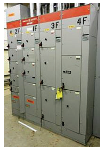
Their motor control center is out of production, making replacement parts hard to find.
